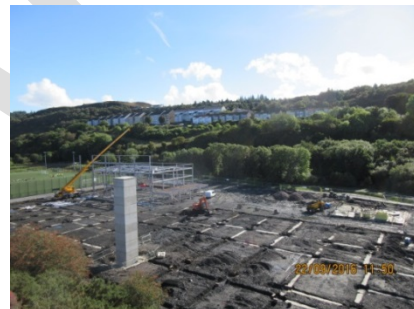
4 High level view of site with Lift Shaft No 1 and Sports Hall Steelwork
